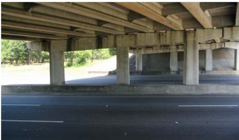
Photo 9: Staining on sides of pier caps
