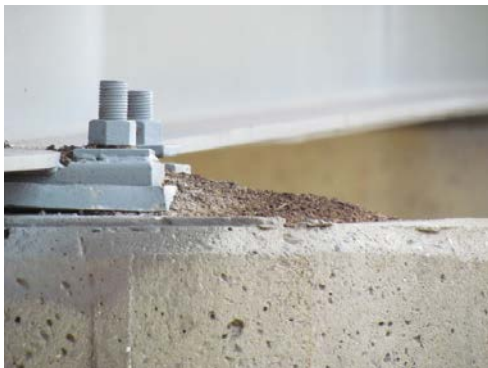
Photo 5: Guano deposit on pier, obscuring structural features.
