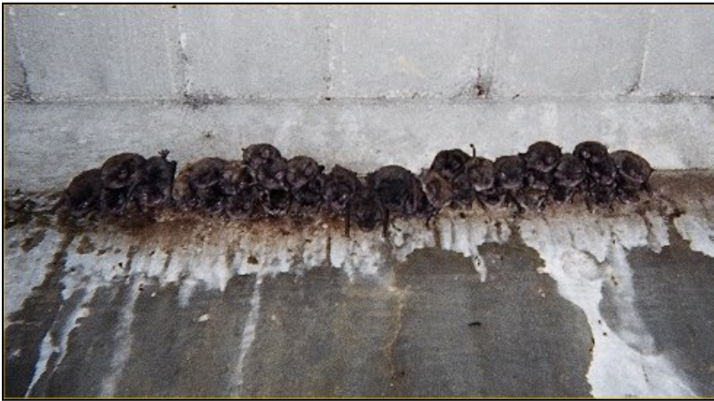
Photo 11: Bats Roosting & Associated Staining
