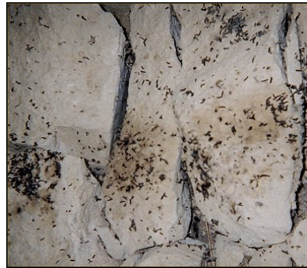
Photo 6: Bat Guano on Riprap
